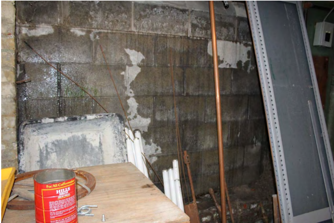
Photo 37. Detail of water leaks along the interior walls in the basement.
