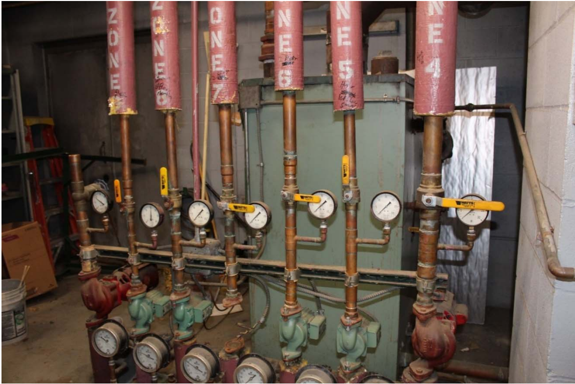
Photo 85. Detail of the boiler in D Block.
