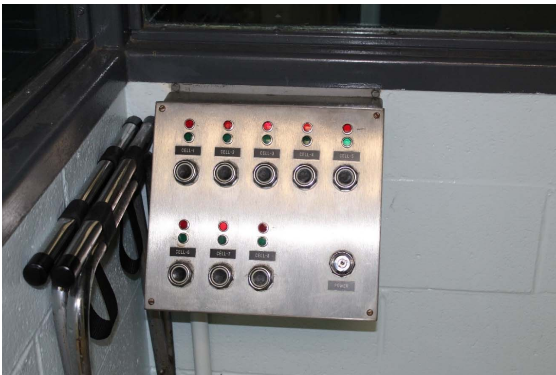
Photo 98. Detail of the D Block cell door controls.
