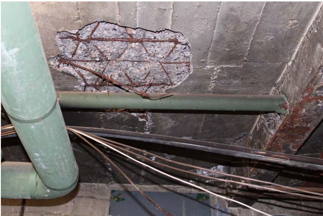
Photo 38. Detail of ceiling erosion in the basement under jail.
