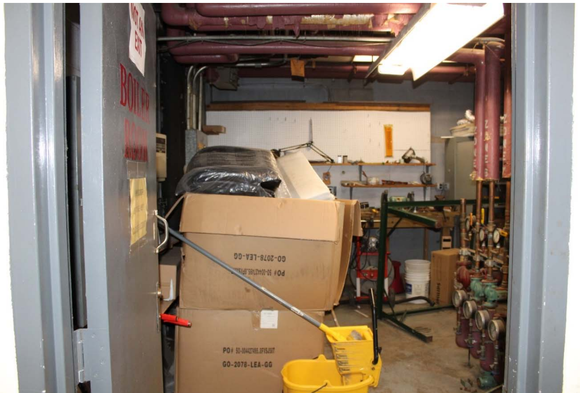
Photo 84. View of the boiler room on northside of D Block.
