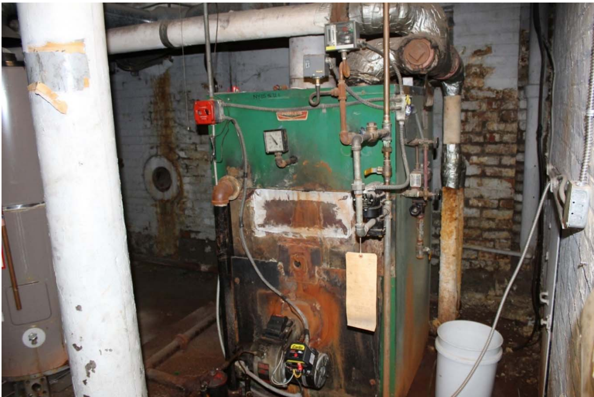
Photo 34. Detail of the basement furnace servicing the jail.
