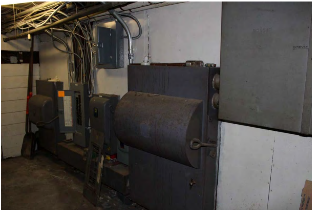
Photo 71. Detail of the original and updated fuse and breaker boxes in the basement of the Sheriff's Offices.
