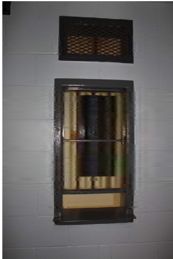
Photo 97. Detail of an access window into the common area of D Block.
