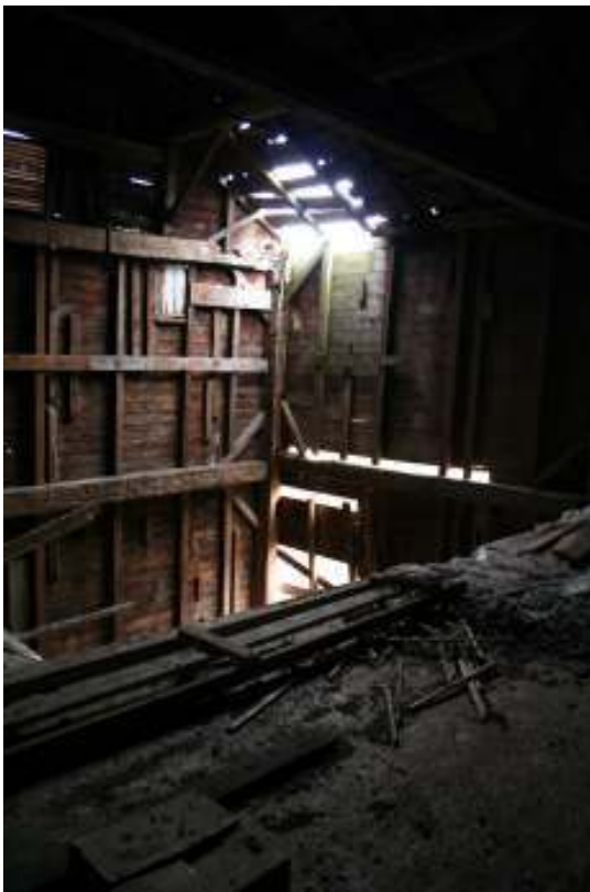
Photo 16. View of the interior northwest corner of the English threshing barn showing hay mow area below and roof damage above, facing northwest.
