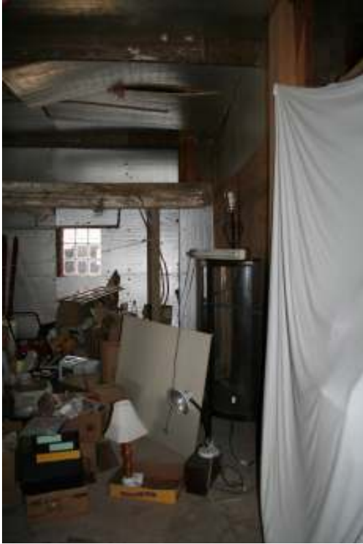
Photo 23. View of Dutch barn ground-level looking at northwest corner where both the sill and end girt are missing, facing west.
